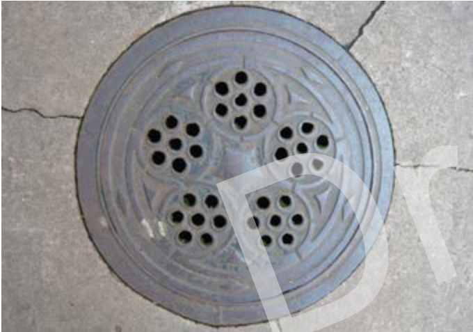
Photo 80: The cast iron coal hole cover outside 101 High Street
