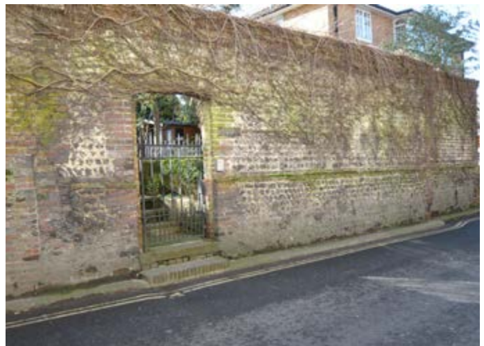
Photo 82: The front garden wall to the Mansion House dates from the 18th century and is Grade II listed
